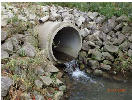
Photo 8. Perched culvert under Sunningdale Road West.
