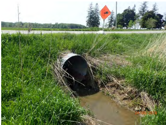
Photo 20. Large CSP under Wonderland Road facing West (June 2018).
