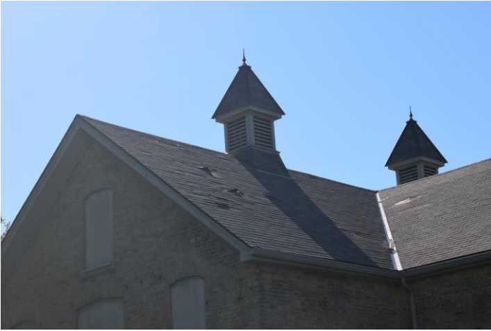
Photo 7: Horse Stable north elevation roof with lifting shingles
