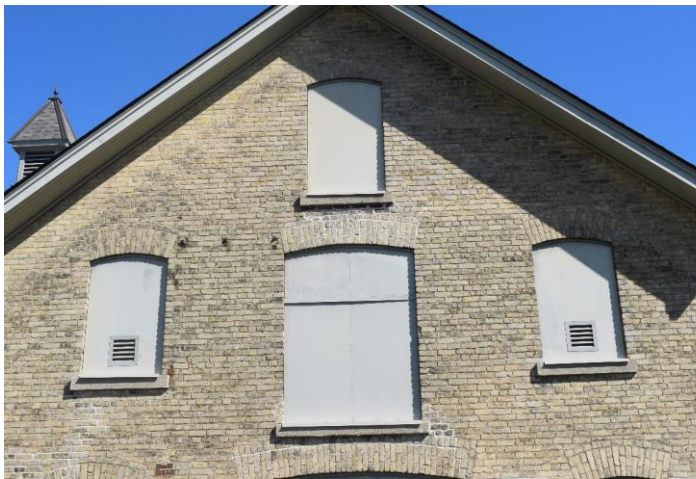
Photo 15: Horse Stable south elevation gable with boarded-up windows with venting
