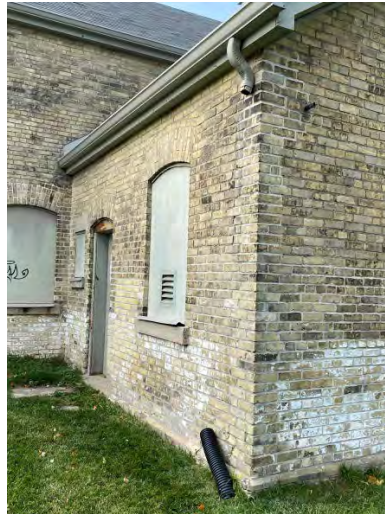
Figure No. 89: South Elevation Missing RWL (Photo No. 12.0)
