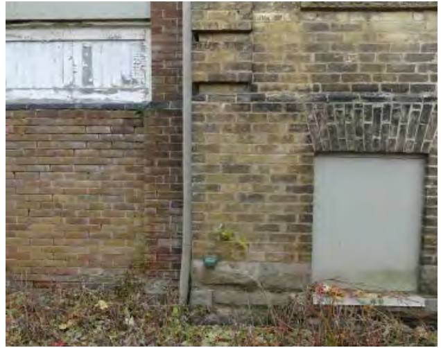
Figure No. 159: East Wing – North Elevation – Wing/Porch Connection – Detail at Grade (Photo No. 62.3)
