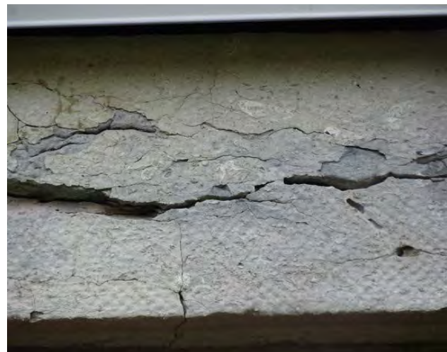
Figure No. 322: East Elevation Cracked Sill Detail (Photo No. 19.9)
