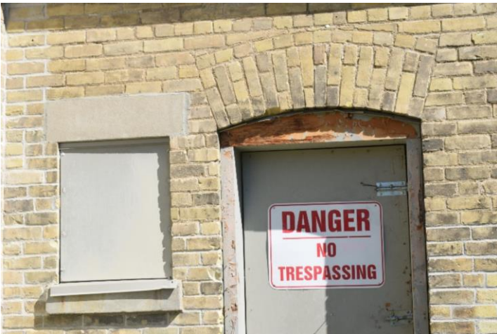
Photo 11: Horse Stable close-up of brick voussoir above entry door and window sill and lintel
