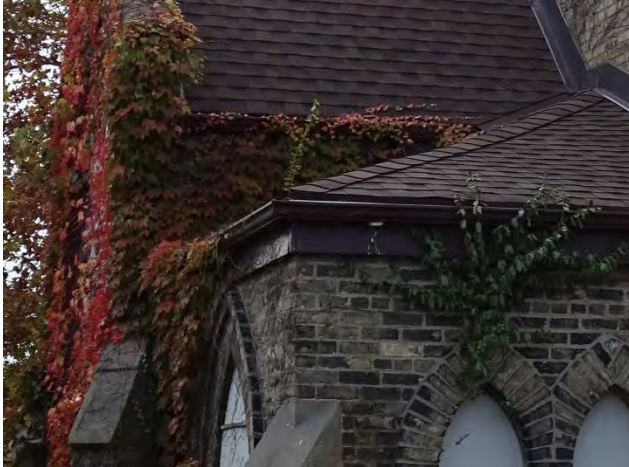
Figure No. 20: North Elevation – Sanctuary Gutter (Photo No. 13.4)
