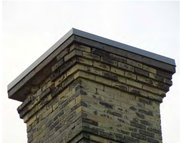
Figure No. 175: East Wing – Stair Tower Chimney – South Elevation Detail (Photo No. 74.4)
