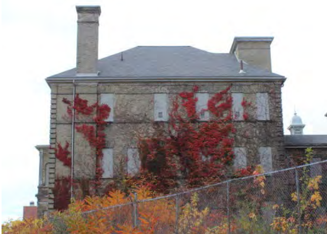
Figure No. 168: Central Administration Block –South East Chimney – East Elevation (Photo No. 71.0)
