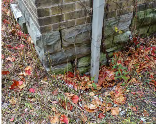
Figure No. 221: West Wing – South of West Corridor – East Elevation (Photo No. 97.0)
