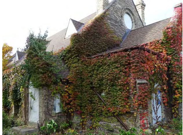
Figure No. 21: South Elevation – South Entrance Wing Gutter and Broken RWL (Photo No. 15.4)
