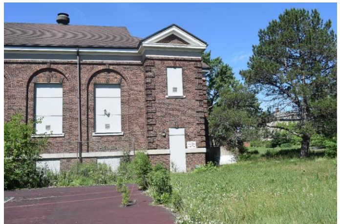
Photo 64: Recreation Hall east elevation boarded-up window and door on projecting bay
