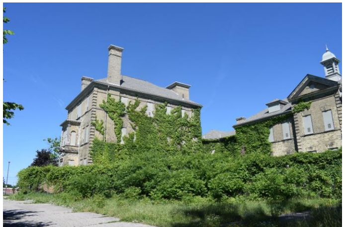
Photo 28: Infirmary southeast elevation of Administration Block and part of south elevation of east wing
