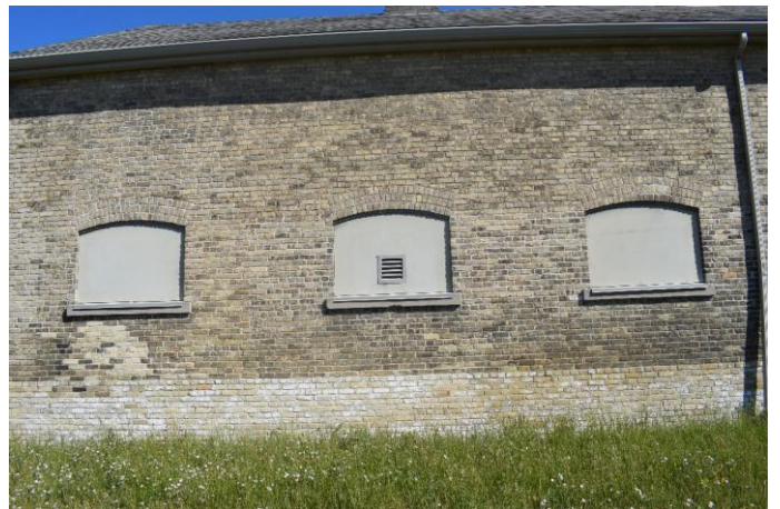
Photo 16: Horse Stable south elevation boarded-up windows with venting
