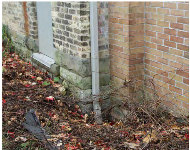
Figure No. 161: West Wing – North Elevation – West Wing/Porch Connection – Detail at Grade (Photo No. 66.4)
