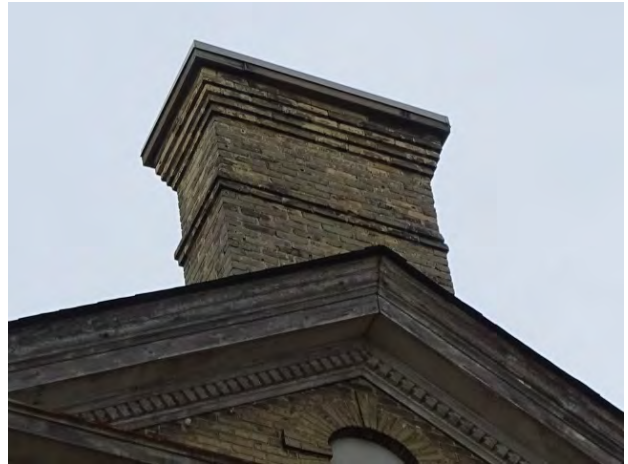
Figure No. 167: Central Administration Block – West Chimney – West Elevation Detail (Photo No. 70.3)
