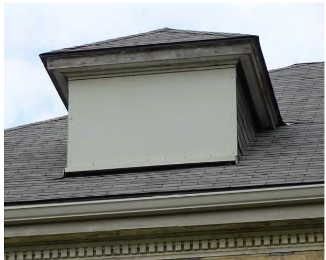
Figure No. 181: West Wing – South Elevation – South West Dormer Detail (Photo No. 77.5)
