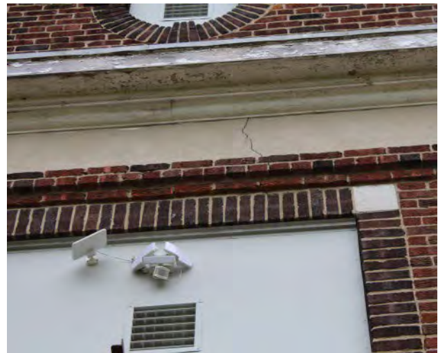
Figure No. 290: North Elevation Frontispiece Crack Detail (Photo No. 9.1)
