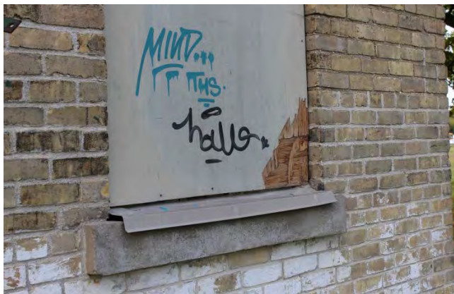
Figure No. 117: Damaged Window Protection (Photo No. 24.13)
