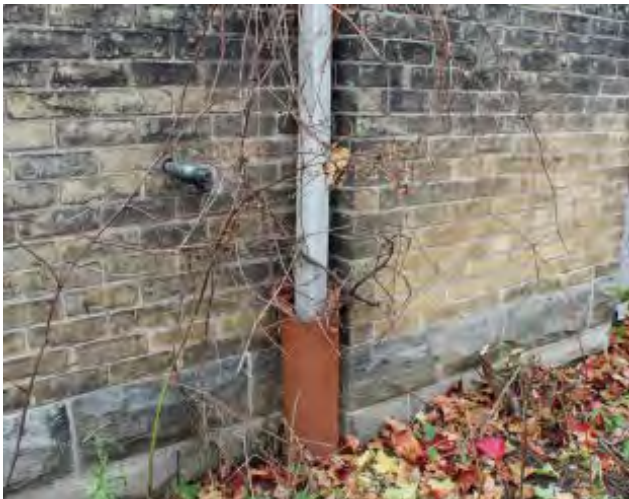
Figure No. 154: Central Administration Block – East Elevation – Detail at Grade (Photo No. 55.1)
