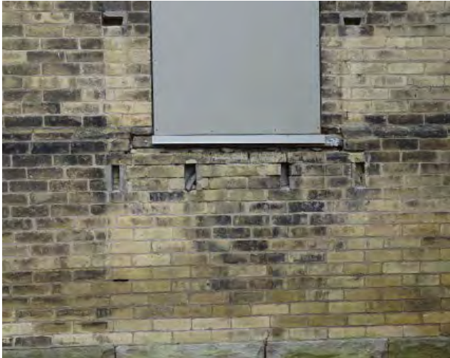
Figure No. 188: Central Pavilion and Corridors – South Corridor – West Elevation (Photo No. 83.1)
