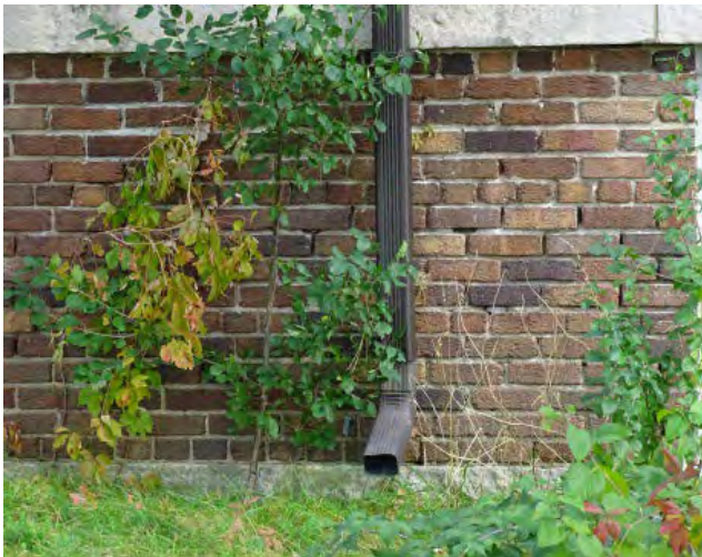
Figure No. 325: West Elevation (Centre) Missing Mortar (Photo No. 21.1)
