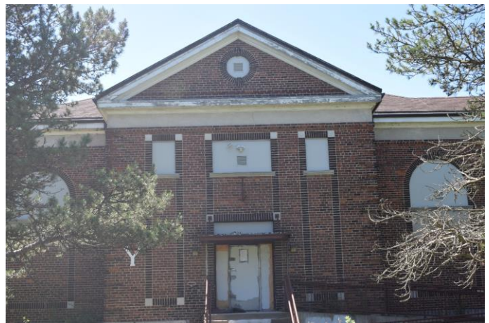
Photo 60: Recreation Hall front elevation boarded-up windows
