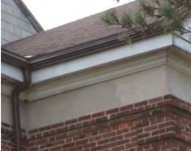
Figure No. 291: North Elevation – Frontispiece East Wing Return Roof Element (Photo No. 9.3)
