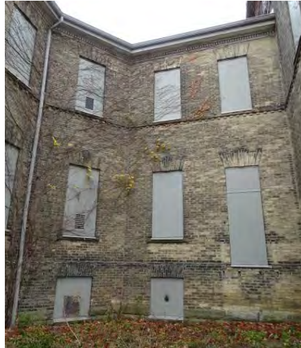
Figure No. 189: Central Pavilion and Corridors – South Corridor – West Elevation (Photo No. 83.0)
