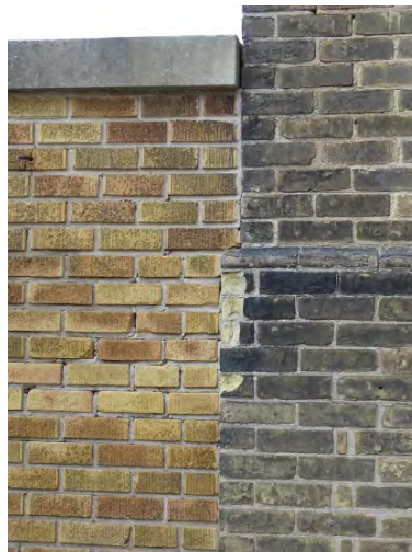
Figure No. 185: Central Administration Block – Entrance – East Elevation – Connection Detail at Stair Addition (Photo No. 80.5)
