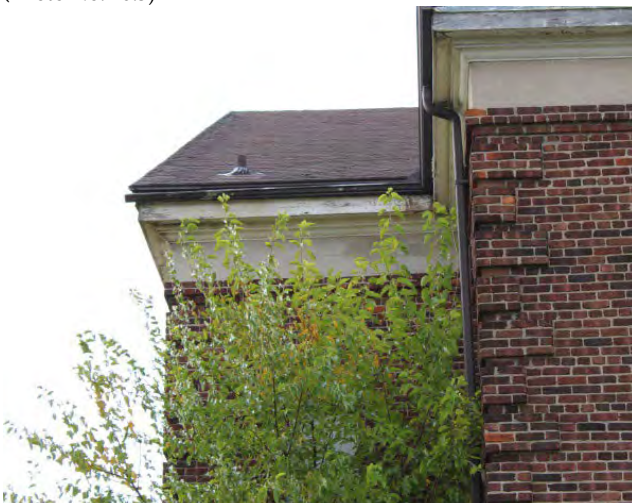
Figure No. 295: East Elevation Main Roof South of Rear East Wing (Photo No. 10.7)
