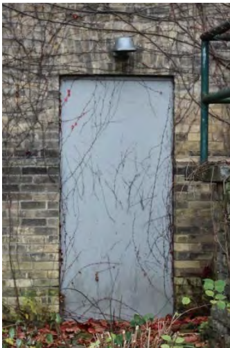
Figure No. 266: Central Pavilion and Corridors – East Corridor – North Elevation – D4-N (Photo No. 104.4)
