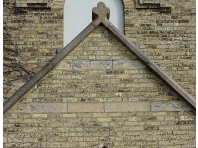
Figure No. 51: West Elevation – West/Main Entrance Stone Capping and Stone Band Detail (Photo No. 27.6)
