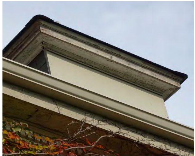
Figure No. 179: East Wing – South Elevation – South West Dormer Detail (Photo No. 76.3)
