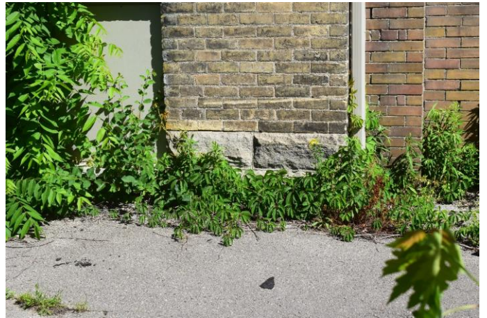
Photo 52: Infirmary close-up of vegetation over foundation
