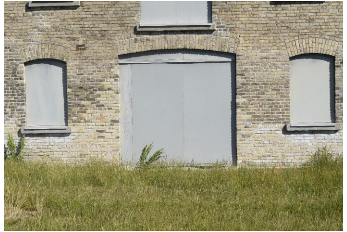
Photo 14: Horse Stable south elevation boarded-up entry door and windows
