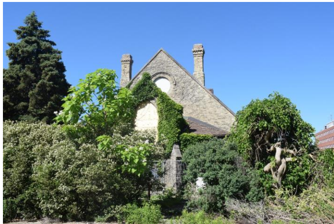
Photo 20: Chapel of Hope rear elevation with vegetation overgrowth, looking west
