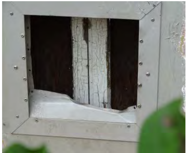
Figure No. 259: Missing Vent (Photo No. 106.33)
