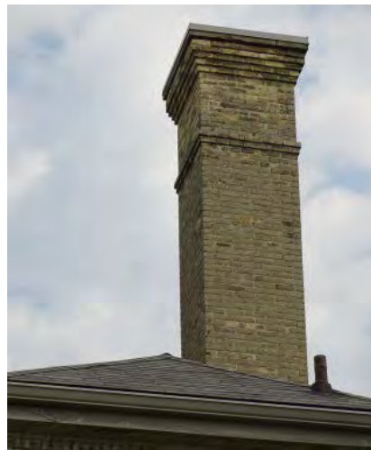
Figure No. 177: West Wing – Stair Tower Chimney – North West Elevation (Photo No. 75.3)
