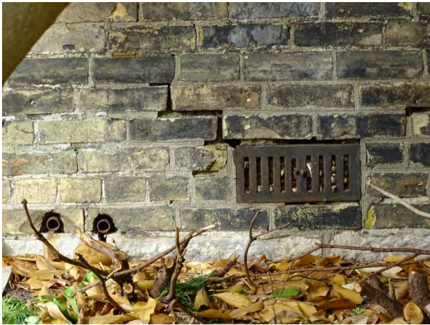
Figure No. 34: South Elevation – Nave – Crack in Brick Wall (Photo No. 22.6)
