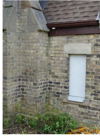
Figure No. 45: East Elevation – North Transept Staining at Grade (Photo No. 21.1)
