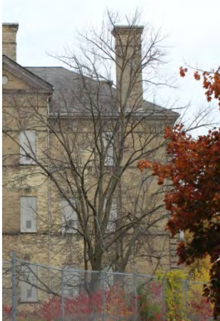
Figure No. 170: Central Administration Block – South West Chimney – West Elevation (Photo No. 72.0)
