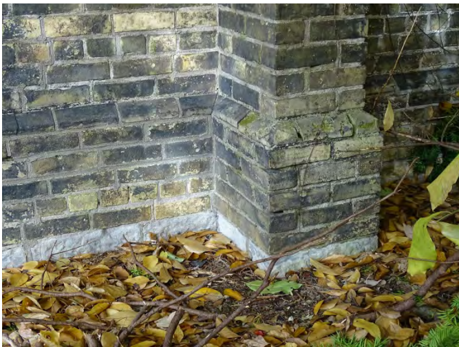
Figure No. 54: South Elevation – Stone Foundation at Nave Wall and Buttress Base (Photo No. 30.1)
