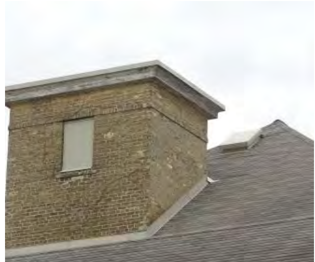
Figure No. 129: Central Administration Block – North West View of Roof (Photo No. 21.1)
