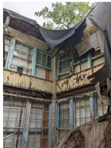
Photo 48: Infirmary east porch roof collapse, photo provided by Old Oak from June 25, 2021
