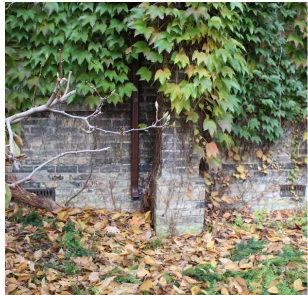
Figure No. 19: South Elevation – Main Roof RWL Detail at Grade (Photo No. 15.3)
