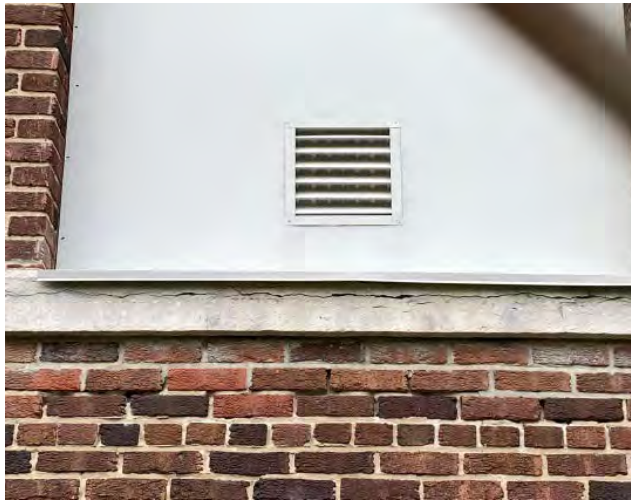
Figure No. 319: East Elevation Cracked Sill (Photo No. 19.5)
