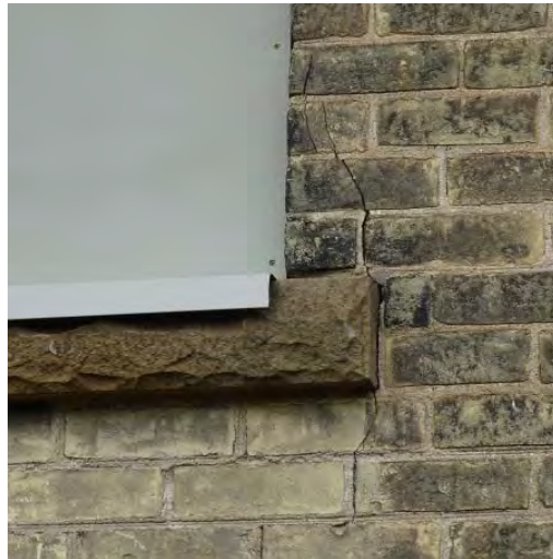
Figure No. 261: Crack at Sill (Photo No. 106.35)
