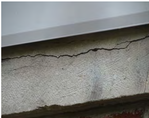
Figure No. 321: East Elevation Cracked Sill Detail (Photo No. 19.8)
