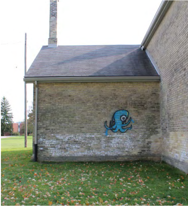
Figure No. 102: Graffiti and White Wash (Photo No. 16.0)
