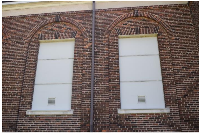
Photo 62: Recreation Hall west elevation boarded-up windows with venting
