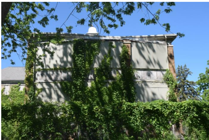
Photo 47: Infirmary east elevation porch end looking northwest prior to porch collapse
