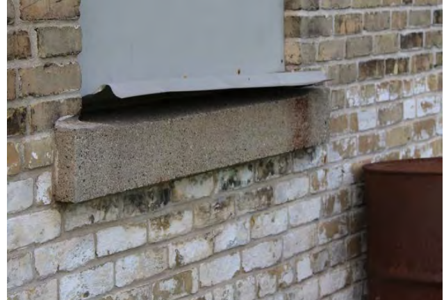
Figure No. 116: Damaged Sill Protection (Photo No. 24.12)
