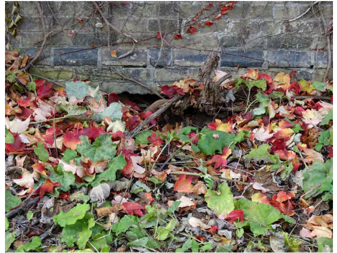
Figure No. 53: East Elevation – Sanctuary Missing Foundation Detail (Photo No. 29.1)
