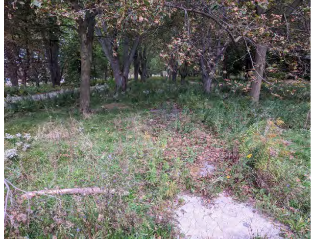
Figure No. 374: View to north of central concrete walkway, poor condition (Photo No. 7.3)
