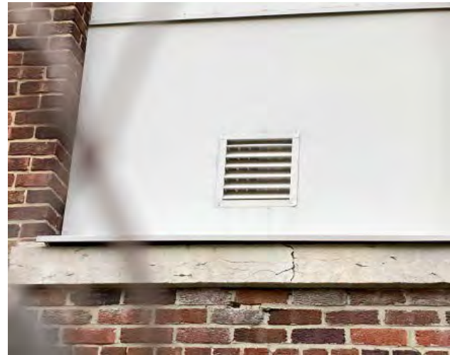
Figure No. 320: East Elevation Cracked Sill (Photo No. 19.6)
