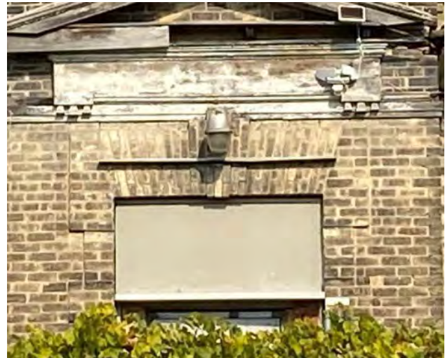
Figure No. 263: Central Administration Block – Entrance – South Elevation – D1-S Transom (Photo No. 107.1)
