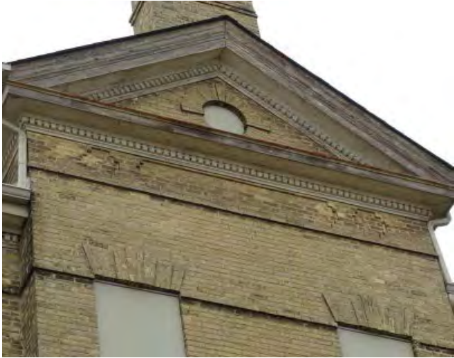
Figure No. 142: Central Administration Block – West Elevation – West Pediment Detail (Photo No. 40.1)
