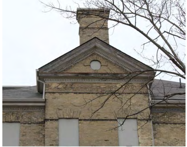
Figure No. 157: Central Administration Block – West Elevation – Leaders from West Pediment (Photo No. 57.1)
