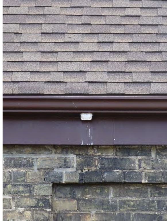
Figure No. 17: North Elevation – Main Roof Gutter and Missing RWL (Photo No. 13.0)
