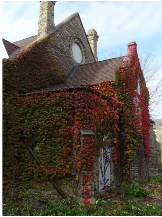
Figure No. 9: East Elevation – Sanctuary and South Entrance Wing Roof Shingles (Photo No. 6.1)
