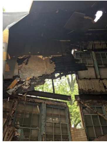
Photo 50: Infirmary east porch roof collapse photo provided by Old Oak from June 25, 2021
