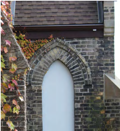
Figure No. 24: North Elevation – West/Main Entrance Gutter and missing RWL (Photo No. 13.6)
