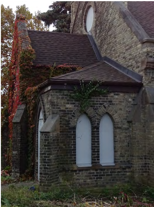
Figure No. 8: East Elevation – Sanctuary and North Entrance Wing Roof Shingles (Photo No. 6.0)
