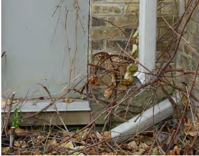
Figure No. 156: Central Administration Block – Entrance – East Elevation – Detail at Grade (Photo No. 56.2)
