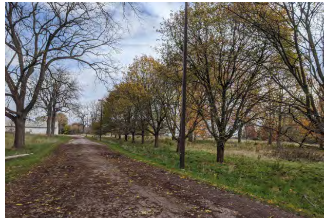
Figure No. 356: View to east along Section 3, failed asphalt paving, grass roadside shoulders and ditches (Photo No. 2.2)
