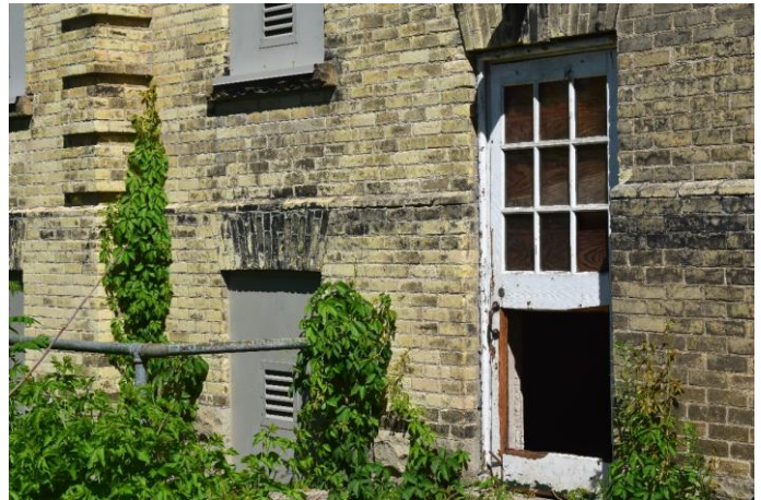
Photo 46: Infirmary kicked-in original door on south elevation
