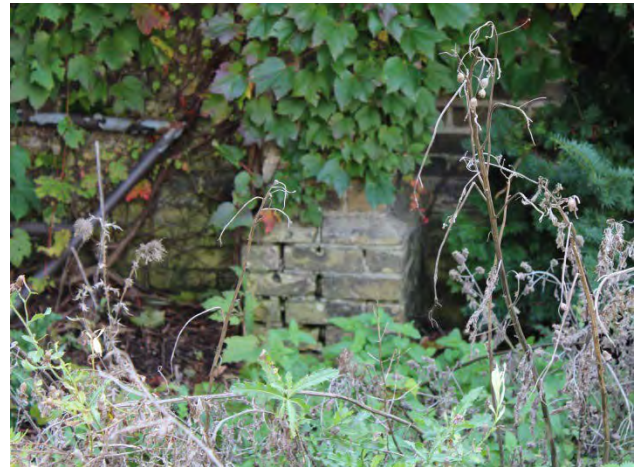
Figure No. 35: South Elevation – Nave Detail at Base of Buttress (Photo No. 22.10)
