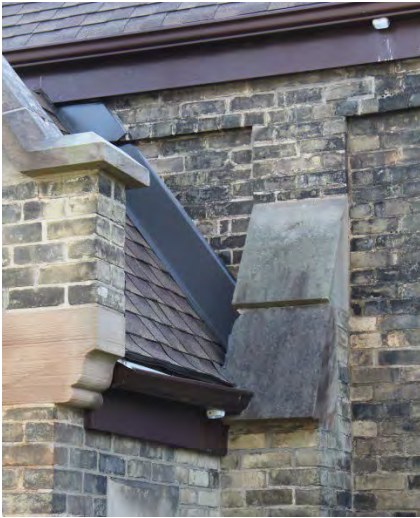
Figure No. 22: West Elevation – North Transept Gutter and Missing RWL (Photo No. 16.0)
