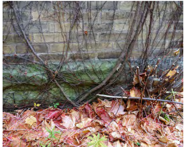
Figure No. 211: East Wing – South of East Corridor – West Elevation (Photo No. 95.0)
