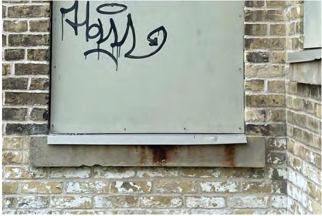
Figure No. 115: Stained Stone Sill (Photo No. 24.11)
