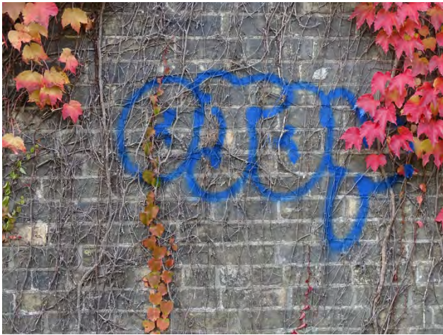
Figure No. 40: East Elevation – Sanctuary Graffiti (Photo No. 21.9)
