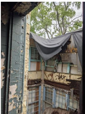
Photo 14: East porch collapse in June 2021
