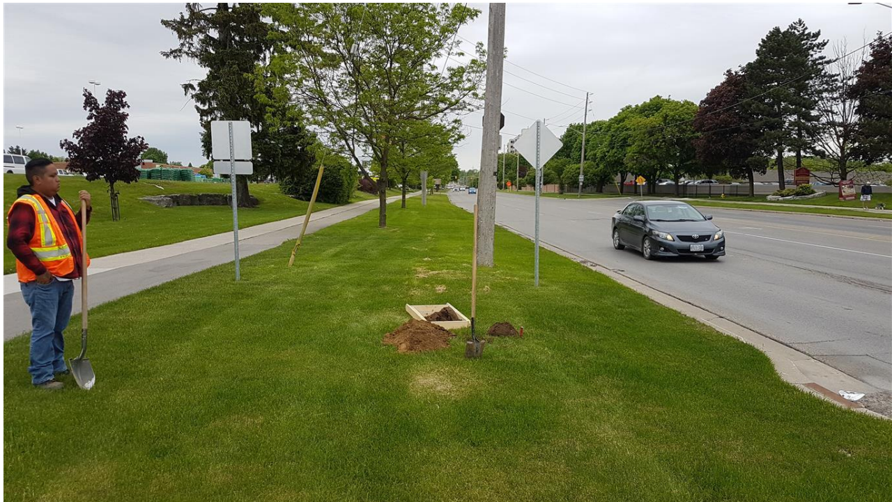
Image 19: Test pitting; facing northwest at the northwest corner of Adelaide Street and Fanshawe Park Road, June 4, 2019.
