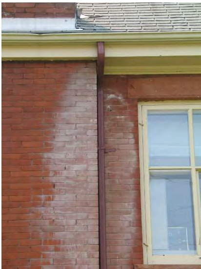
521 Colborne St.– Water Damage
