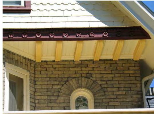
298A Wolfe St. – Soffit & Window
