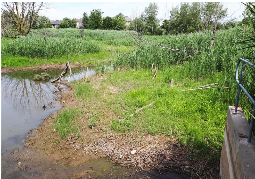
Figure 8: View north northwest from the west side of the culvert. Note the reeds, pond, and undeveloped land (July 20, 2018).
