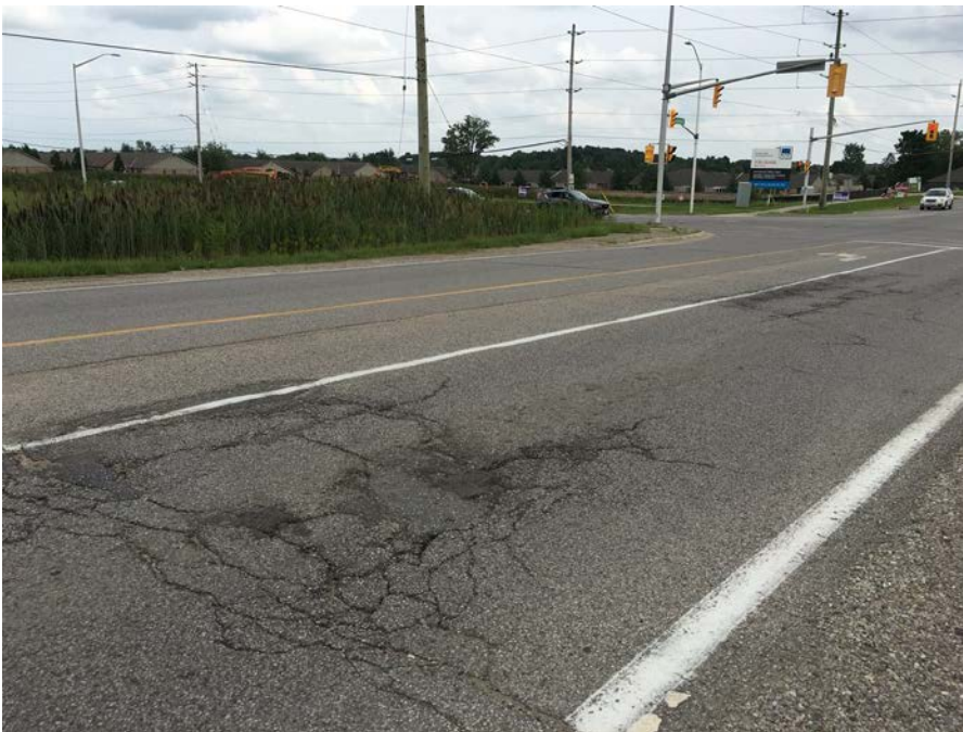
Photograph 2: Adelaide Street North looking southeast at Sunningdale Road East. Note cracking and patching.
