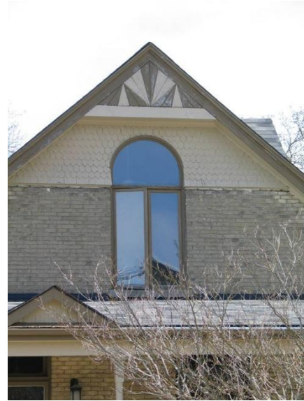
Image 19 - Window alteration, 67 Cathcart, modern intervention in sympathetic style
