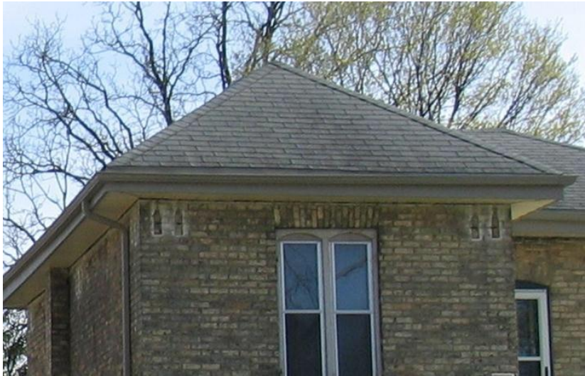
Image 34 - Missing brackets, 27 Askin
